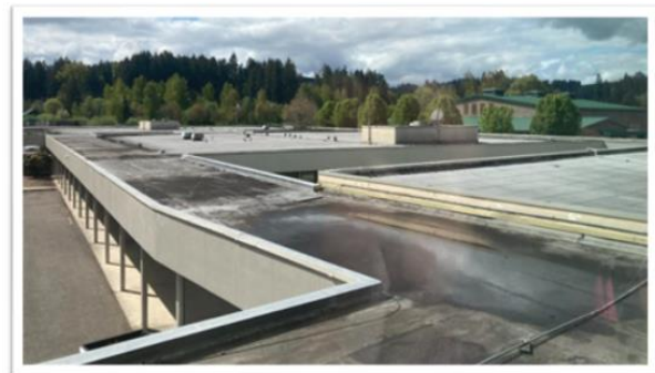
Most classroom sections of SHHS were built as economically as possible before school security was a concern with flat roof construction and are nearing the end of their lifespan.
