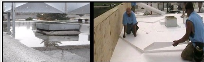
Install a tapered slope insulated roof panel system to the junior high's flat roof. This will provide sufficient slope for water to drain and stay out of the building instead of forming puddles in low spots causing leaks and water damage.
