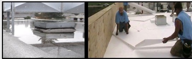
Install a tapered slope insulated roof panel system to the junior high's flat roof. This will provide sufficient slope for water to drain and stay out of the building instead of forming puddles in low spots causing leaks and water damage.
